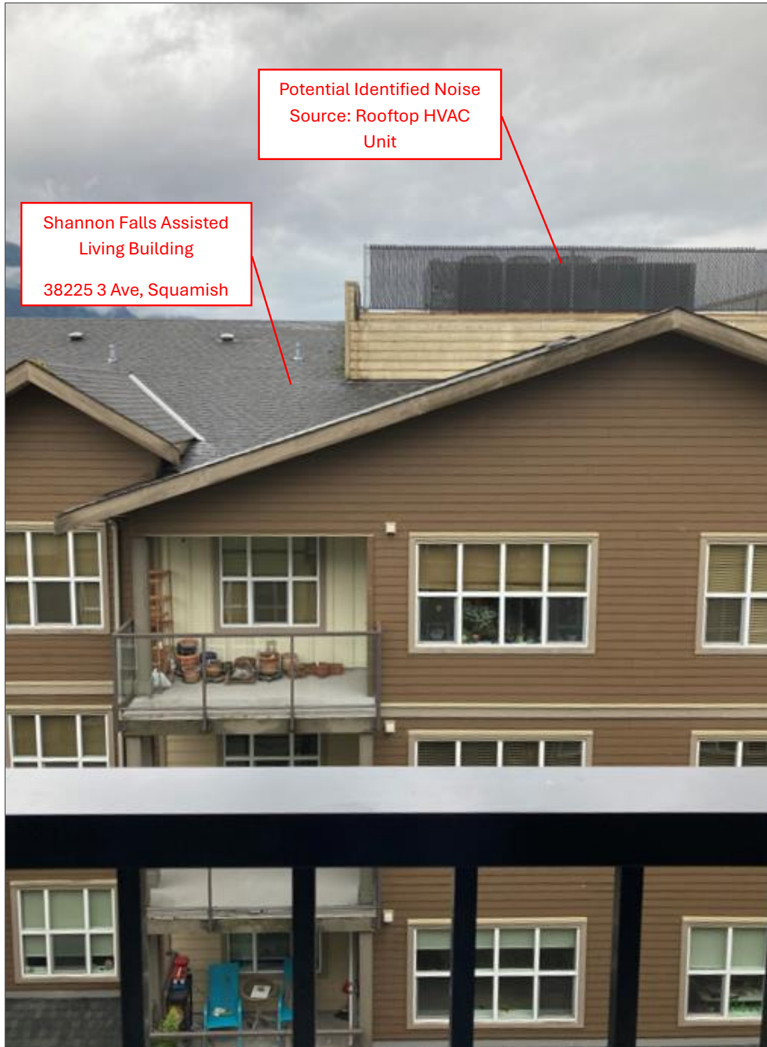
Figure 2 – View of neighbouring rooftop HVAC unit atop the Shannon Falls Residential Building from the balcony of WestWinds Unit 514.
